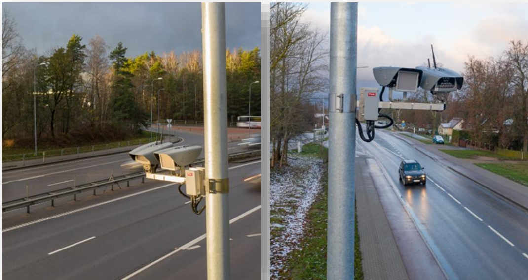
Figure 1. Traffipax LLC, Pole Mounted Camera and Speed Measurement Device.
